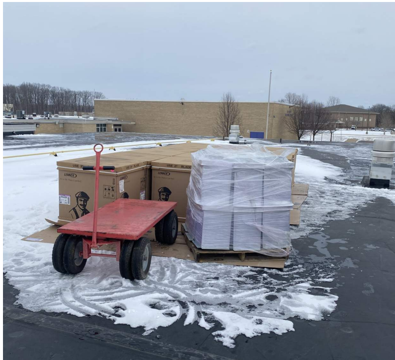
Boxed condensing units on the roof.
