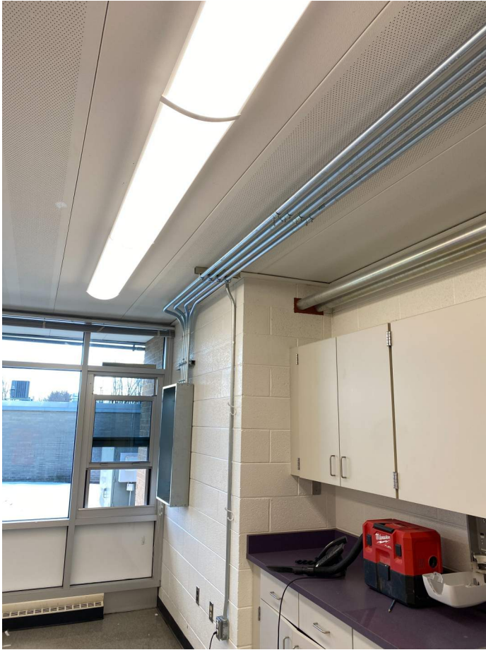
Ceiling view of raceways to panel.
