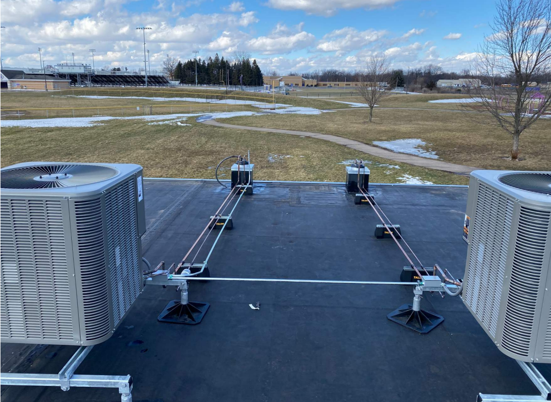
Rooftop condensers and piping.
