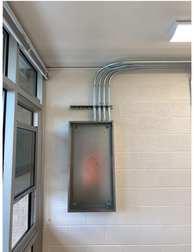
Front view of raceways to panel.
