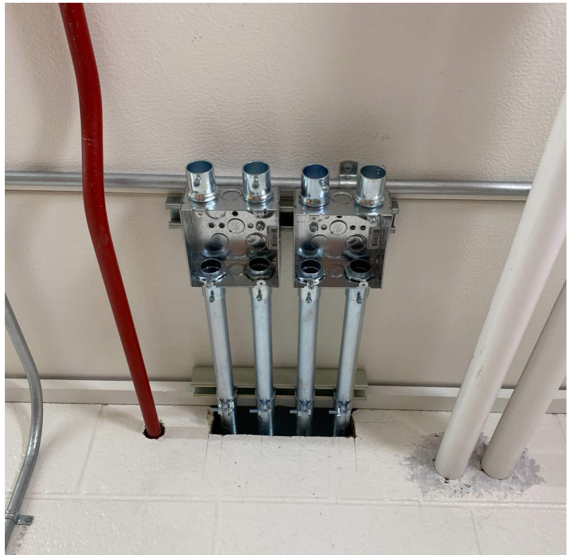
Raceway penetration through wall prior to fire caulk install.
