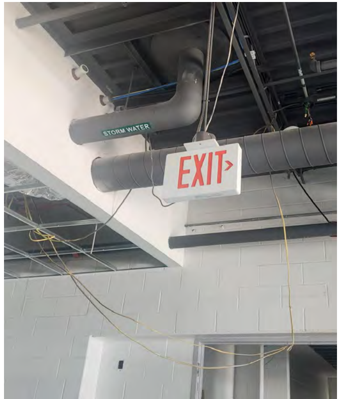
Exit sign installed.
